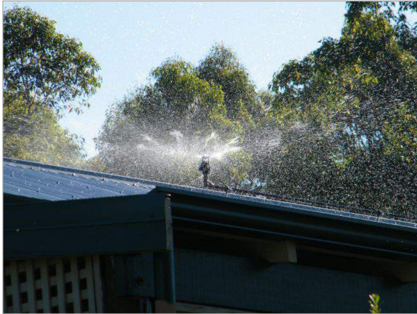
Figure 3. Example of a sprinkler used on a rooftop to protect the building from ember showers. Photo credit: Small Farm Services, Australia.
